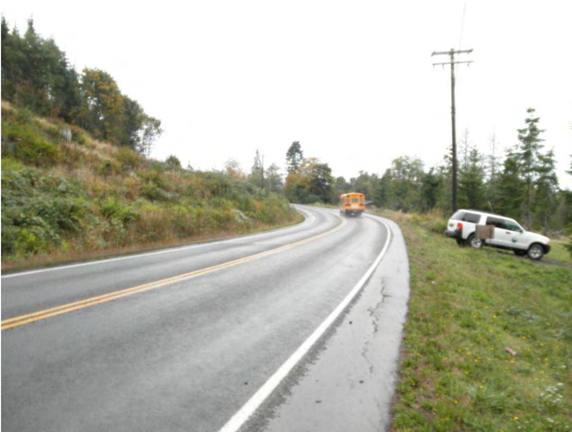
Curve northerly of County Road shop with a.m. shade in winter Elochoman Valley Road, approx. m.p. 0.5
